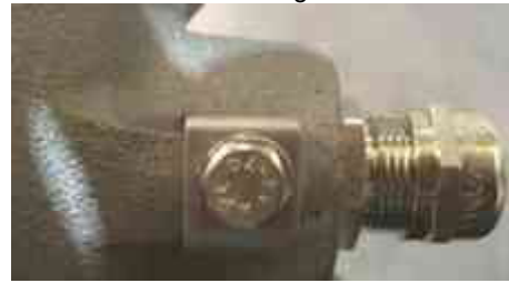
External Earthing Terminal
