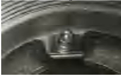
Internal Earthing Terminal
